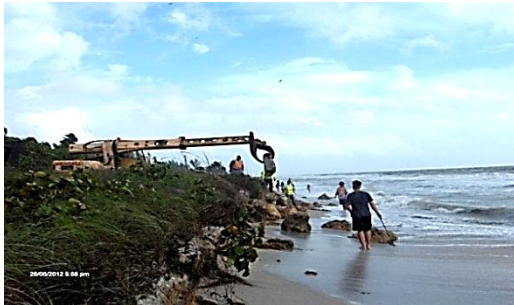
County DOT adds boulders to prevent undermining the road at the curve before Jensen's on the Gulf
