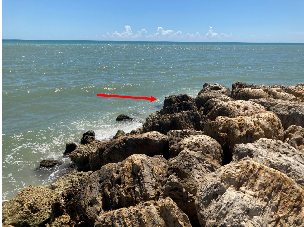
Figure 11. Southwest view of the seaward end of the Blind Pass terminal groin. Note the steep slope in some locations.
