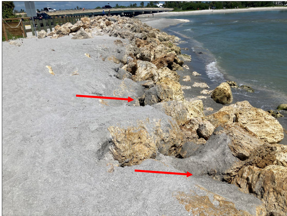
Figure 10. Localized sand loss through or over the structure. There appears to be localized settlement of the stone.
