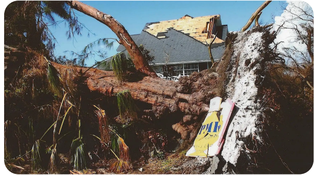
Figure 4. Hurricane Damage on Captiva Island
